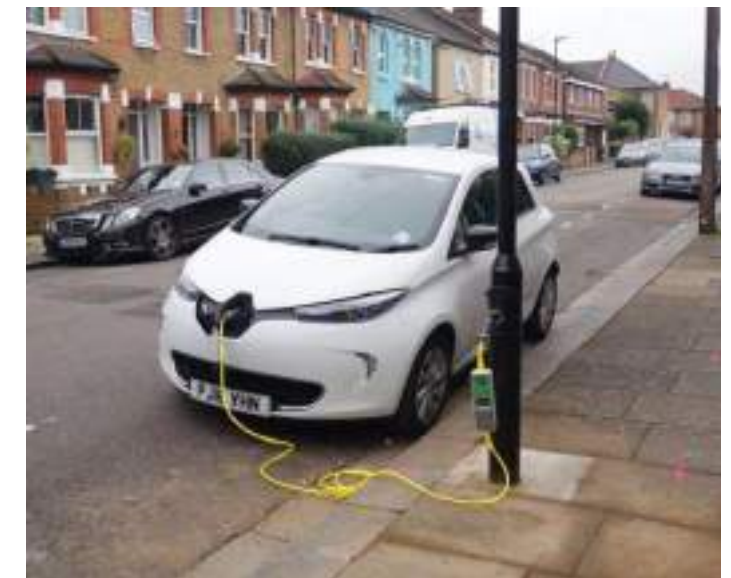
Residential lamp column charging / London
