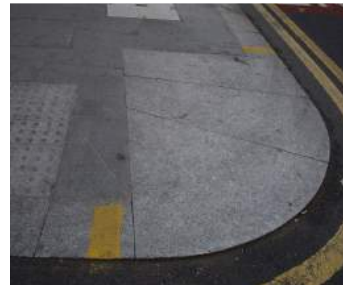
Granite quadrants and 'specials' / improve appearance of kerbline at junctions. Example: Leyton High Road
