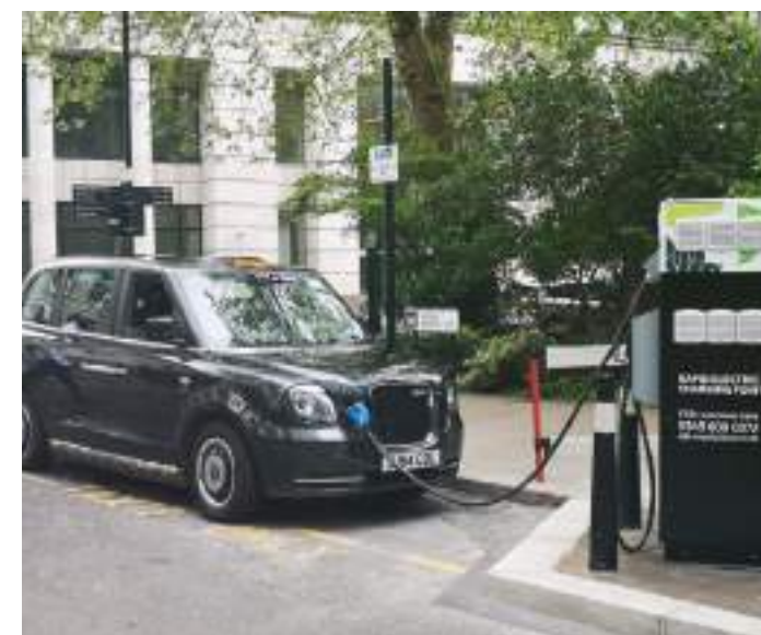
Free-standing rapid charging point / London
