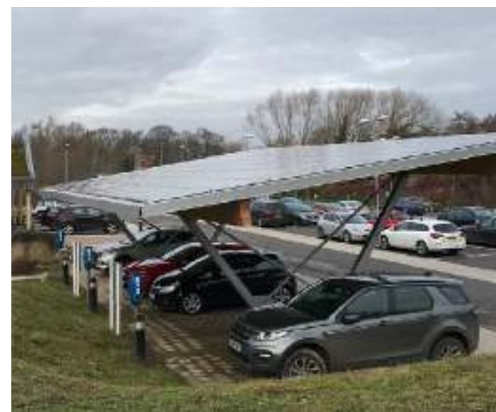
Charging within car parks, using solar
