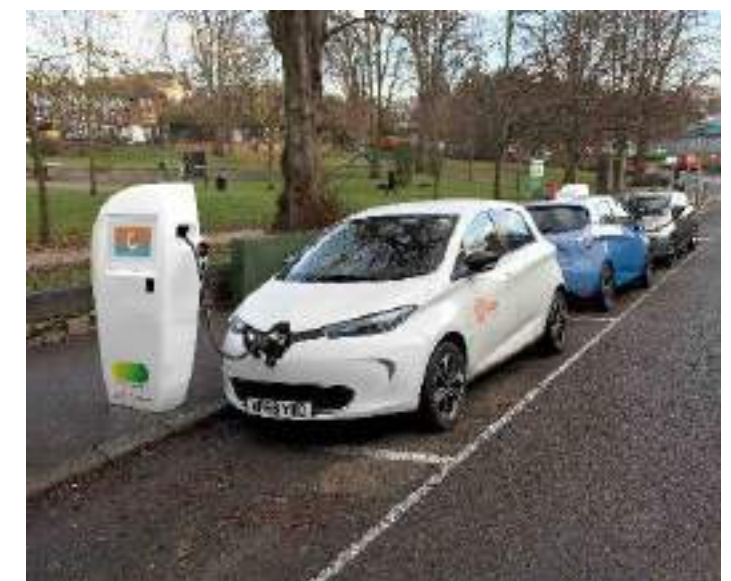
Unacceptable placement of chargers / Devon
