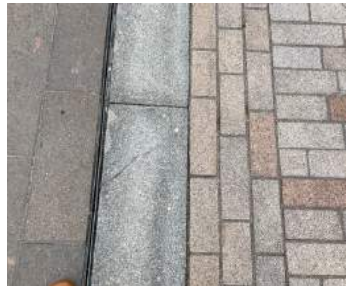
Granite kerb laid flush / 3 courses of setts laid longitudinally emphasizes different footway areas. Example: Kings Cross St Pancras, London
